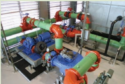
Mechanical room / © William Porter
